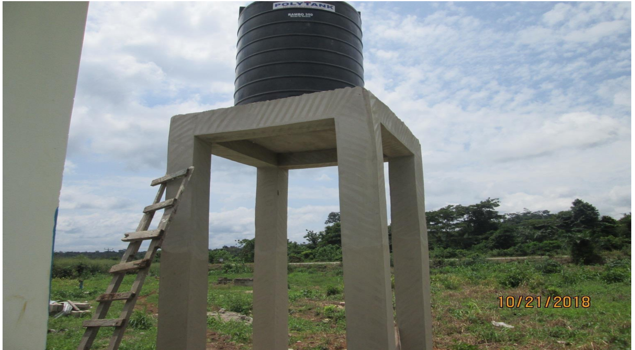
MECHANIZED BOREHOLE ATTACHED TO THE MATERNITY CENTER AT MEHAME, AHAFO ANO SOUTH DISTRICT
