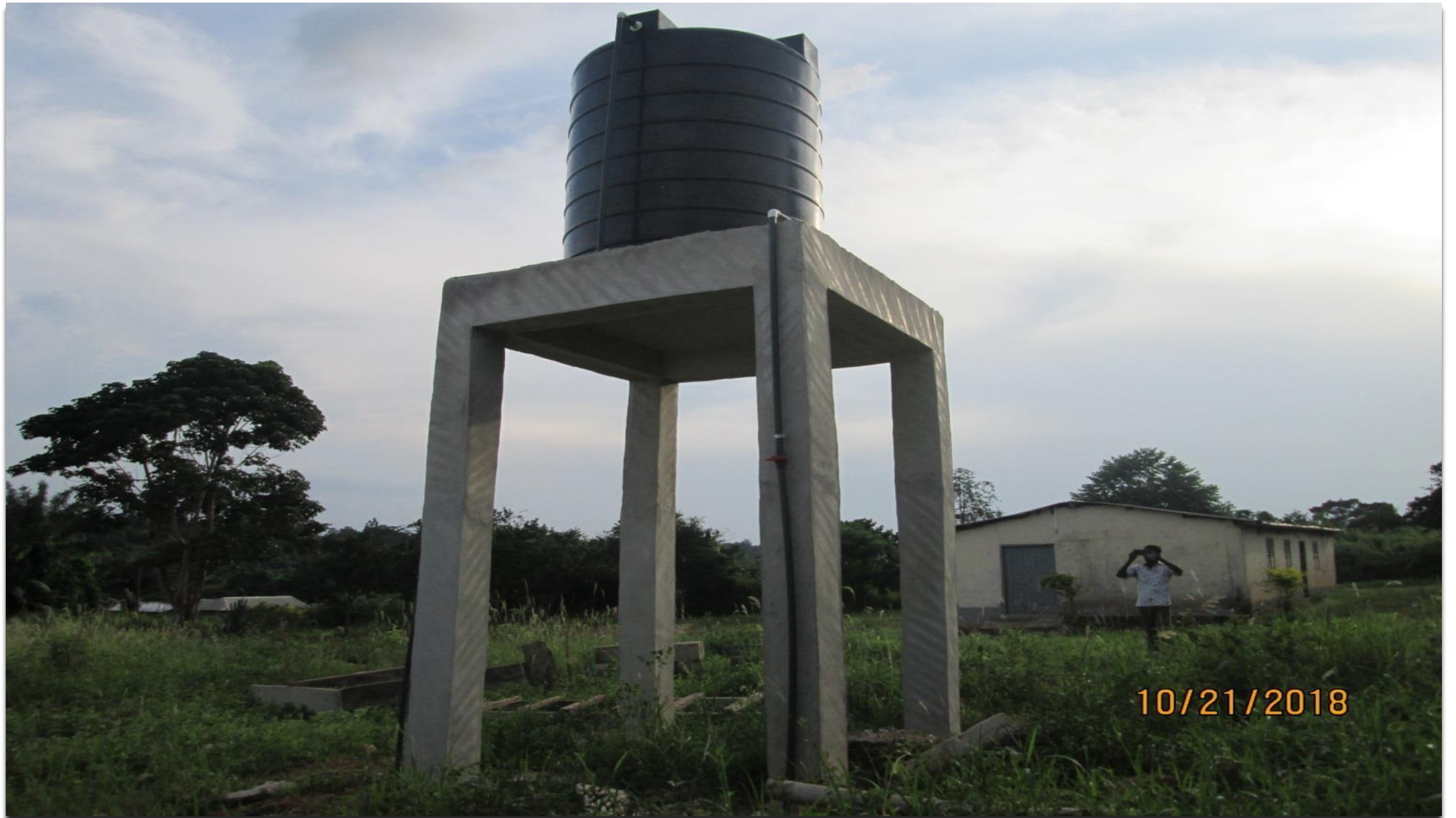
MECHANIZED BOREHOLE ATTACHED TO THE NURSES' QUARTERS AT SABRONUM, AHAFO ANO SOUTH DISTRICT
