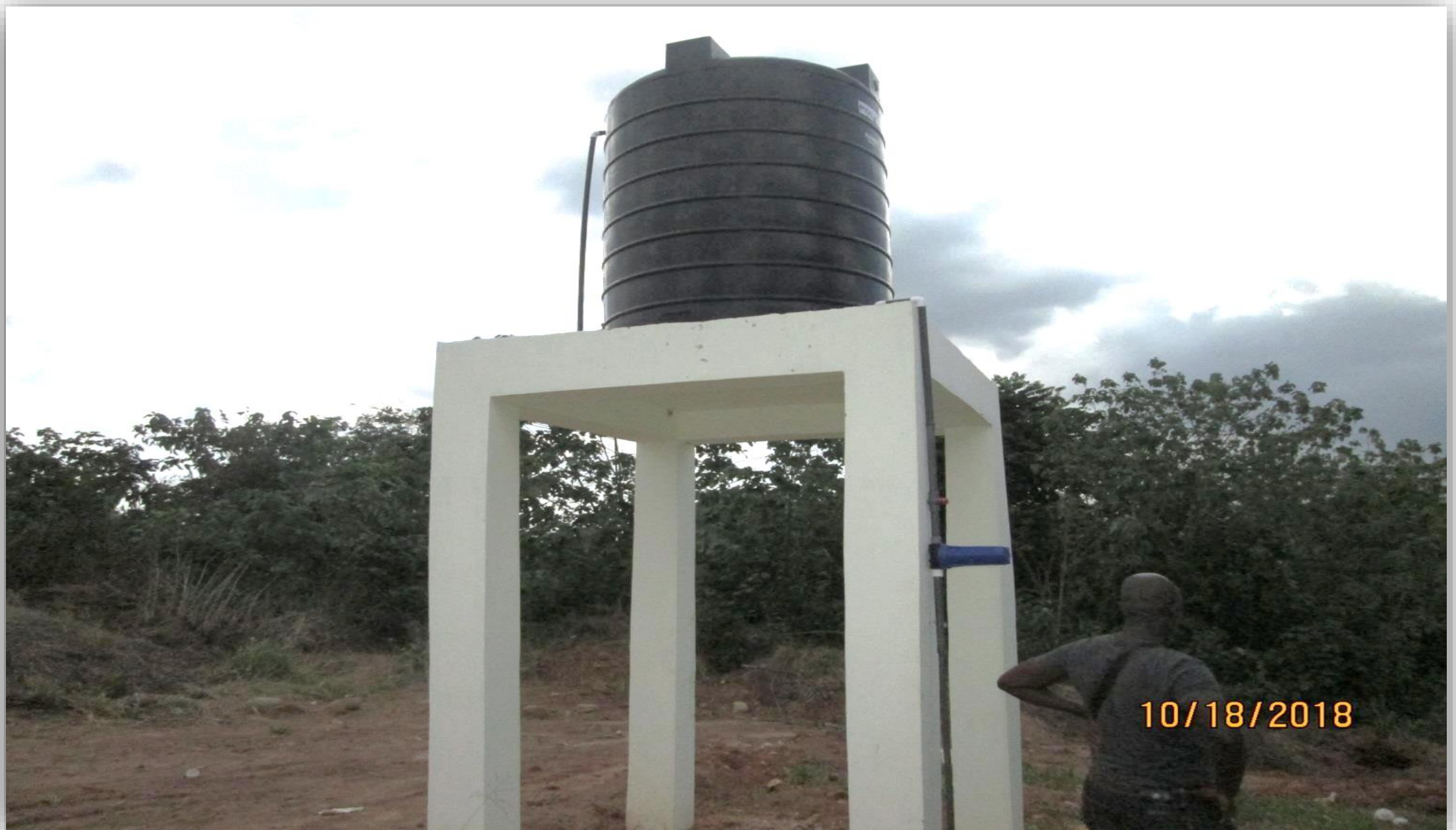
MECHANIZED BOREHOLE ATTACHED TO THE RURAL CLINIC AT NKWANTAKESE, AFIGYA KWABRE DISTRICT
